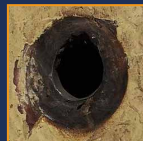
The KOMBO Washer still seals these damaged holes
