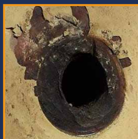
Tight hold prevents hole damage like this
